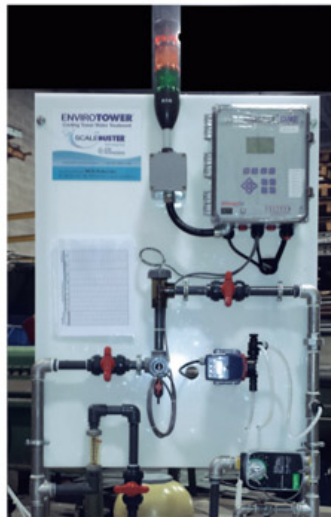
Control Skid Front View
